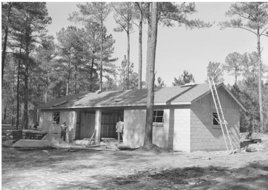
Figure C.6. Workshop, January 1955. The park's new workshop, under construction here, was completed by March 1955. Located near the Senior Ranger's residence, it is still in use as a workshop today. Courtesy, Open Parks Network.
